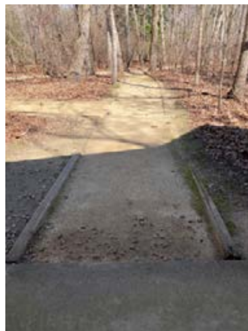
Trails need to be constructed flush at transition area from concrete to gravel
