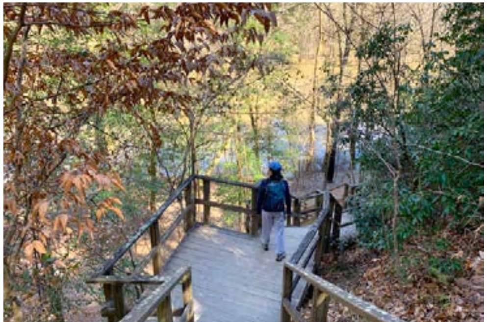
The wooden staircase, that leads to the Cape Fear River, was severely damaged by Hurricane Florence in 2018
