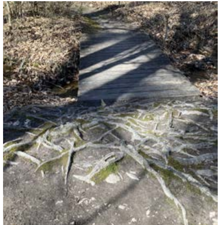
Tree roots along the tributary buffers, have been impacted by park users
