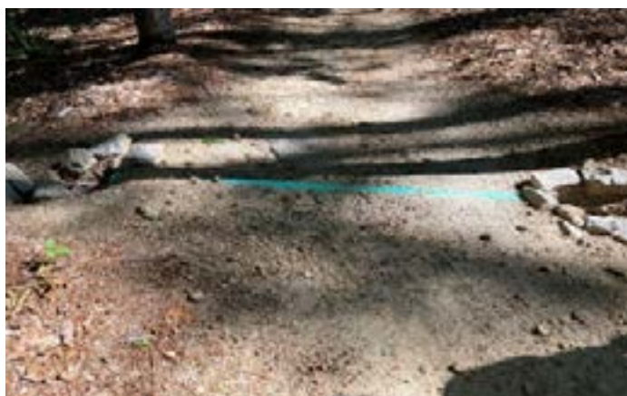
Drainage pipe does not have adequate cover. The impacts from pedestrian traffic will damage the pipe
