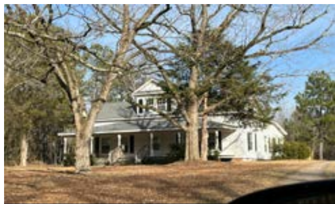
The park residence is over 90 years old and has exceeded the expected lifespan
