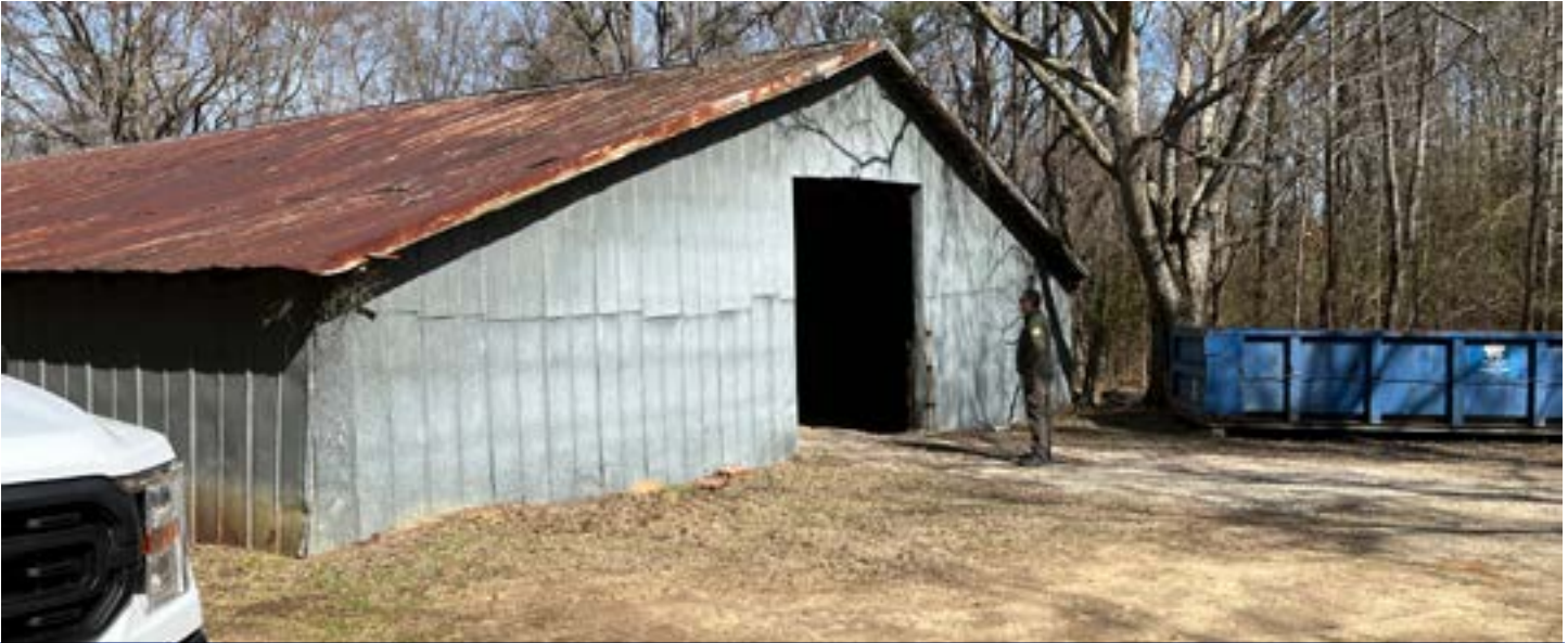
The tin barn needs to be demolished due to age and condition.
