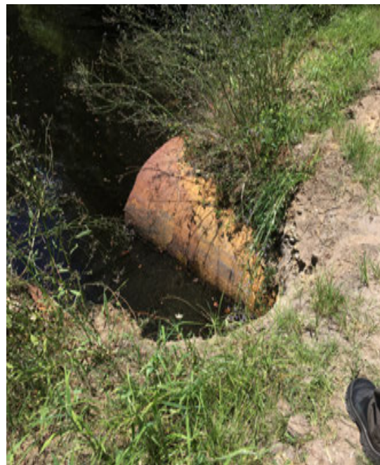
The existing culvert is rusted and cannot adequately divert water
