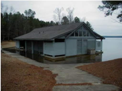
Sandling Beach Shower house No. 1 – Left Side: Bldg. # 040606, 1,131 sq. ft., wood frame, slab on grade. Good condition. Building will flood.
