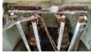
Lift Station - Poor Condition Typical
