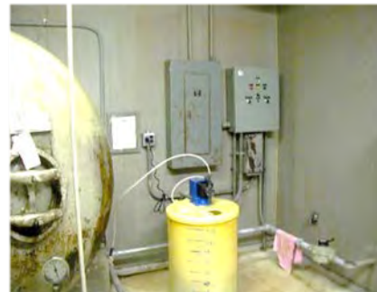
Rolling View Water Control Building: Bldg# 040721, wood frame, 267 sq.ft, inside. Has Corrosion. Built in 1986. Fair condition.
