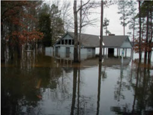
Sandling Beach Shelter No. 4 – Flood Stage: Bldg# 040608, 2,493 sq. ft, wood frame open shelter with toilet inside, in flood stage. Poor condition.
