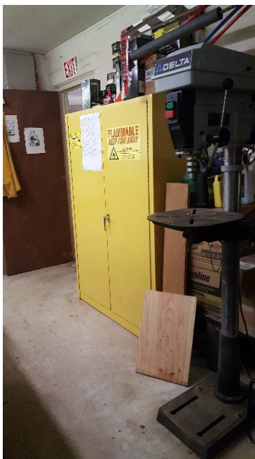
Interior flammable storage area
