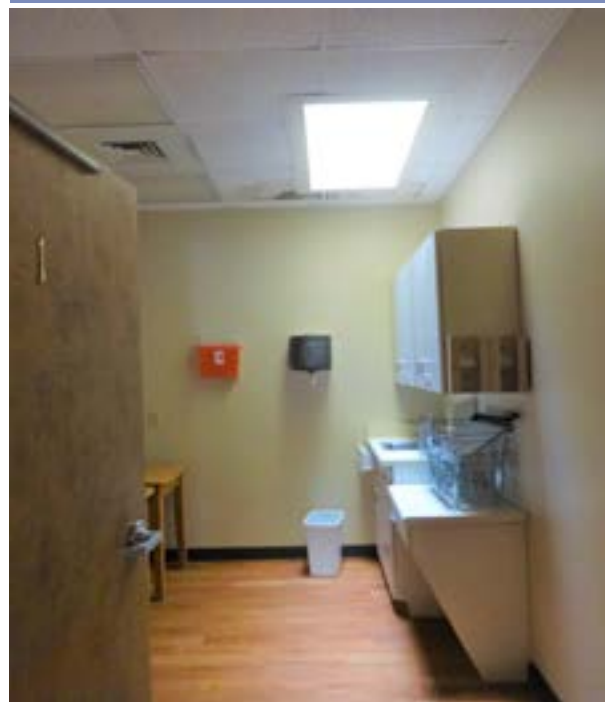
The air conditioning which is located on the roof, leaked onto the ceiling tiles.
