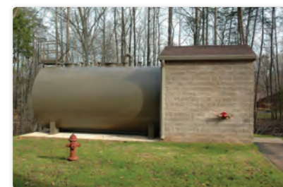
New Sprinkler System.
